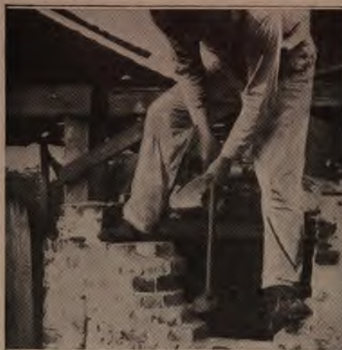
Boiler Tubes Repaired by Driving In Short Pieces of Pipe have Given Service without Trouble for Over One Year
